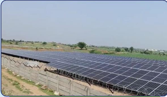
997.50 kWp at Western Metal
