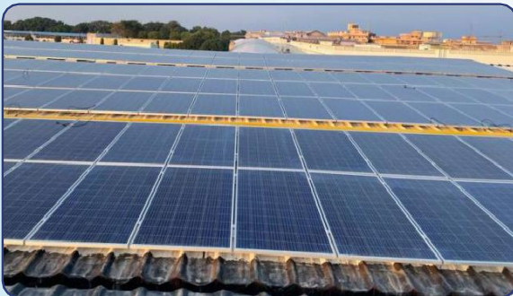
911.2 kWp Solar PV plant at Anandpur Trust , MP
