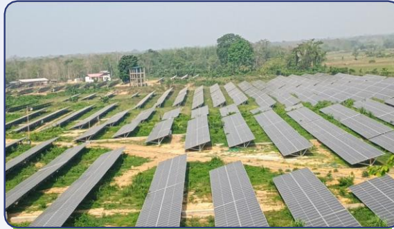
5 MWp at Nagaland Site
