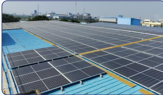
1379.25 kWp at Sumicot Ltd.
